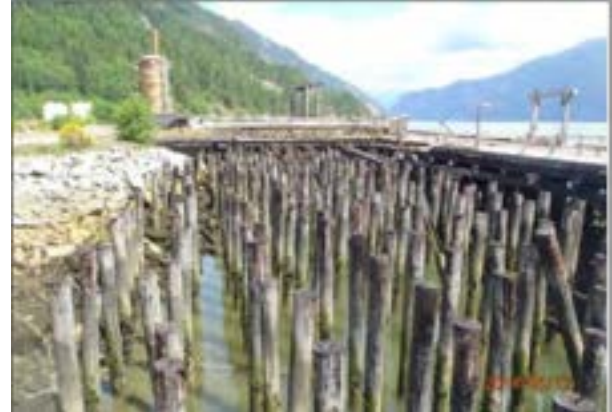
Old marine infrastructure that was removed during restoration Photo by: Keystone Environmental Consultants
